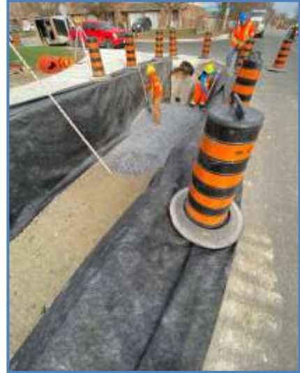
Photo: Hemmingwood Way Bioretention 5
